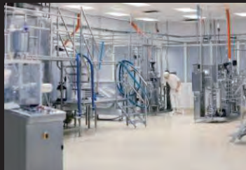
Milk Processing Plant
